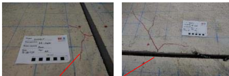
Cracks at the shear connectors
